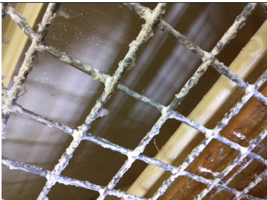
Fig. 3 : first appearance of reddish products below the white oxidation layer after 96 hours of NSS exposure
