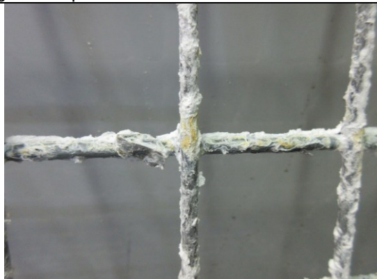
Fig. 7 : Shaped Galvanized Meshes after 240 hours exposure, final rinsing and drying (test end)
